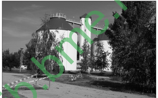
Fig. 4: View of the implemented sludge digesters in Győr
