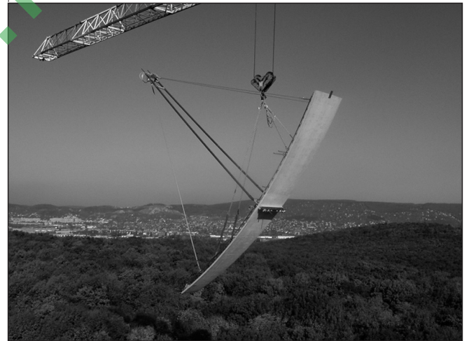
Fig. 7: An individual formwork panel during lifting and after fixing its final position
