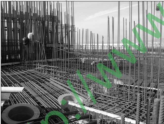
Fig. 6: The reinforcement mesh of the bottom slab and the formwork of the upper slab for the assembly chamber under construction
