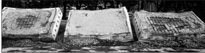
with 1 kg/m 3 polypropylene fibre reinforcement with 3 kg/m 3 polypropylene fibre reinforcement Produced without fibre reinforcement
