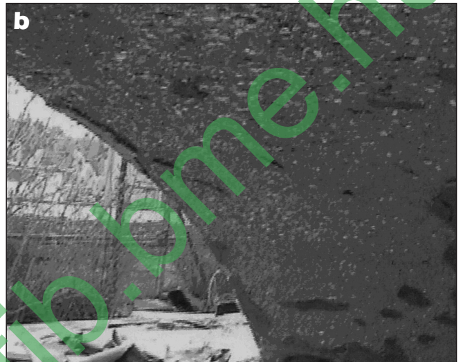
Fig. 3: Tunnel segments after exposure to 1200°C temperature (Mörth, Haberland, Horvath, Mayer, 2005)
