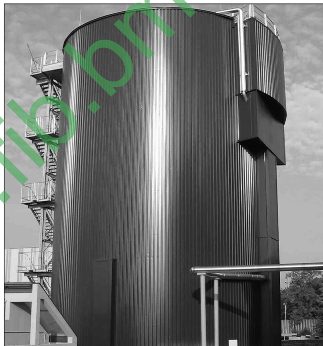
Fig. 8: View of the digester in operation in South-Pest
