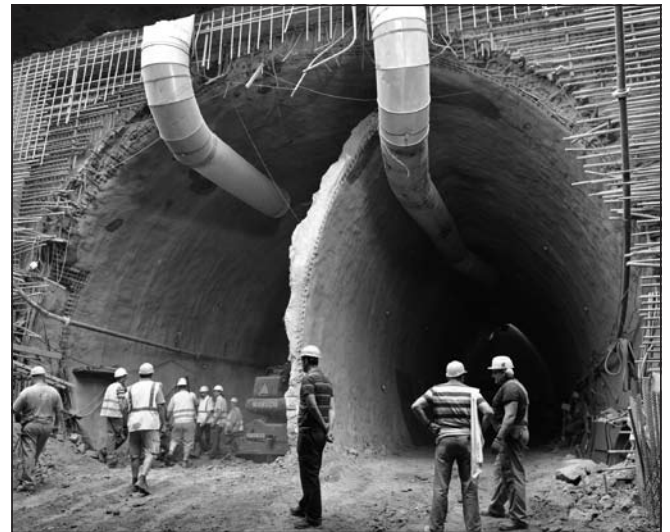
Fig. 12: Construction of SCL tunnel, second phase excavation is ongoing, while the plum kernel shape internal shotcrete lining of the first phase was not yet torn down.
