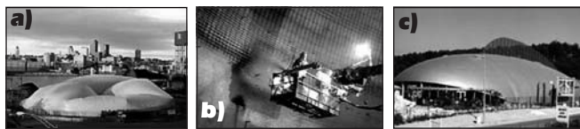
Fig. 28: a) Inflation of formwork; b) shotcreting on the inside of the membrane; c) irregular shape structure constructed with pneumatic formwork (Pirs SA.)
