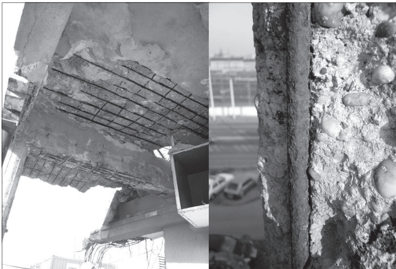
Fig. 3: Spalling of concrete cover and corrosion of steel bars at different structural elements
