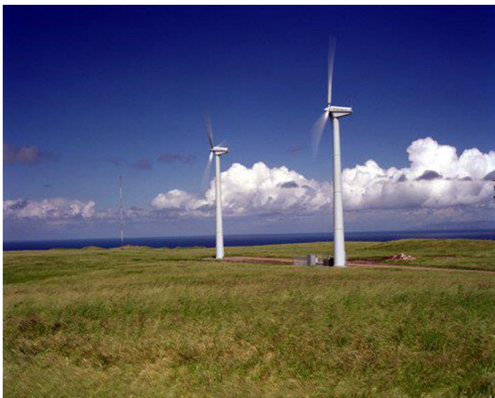
Figure 2: Wind turbines at a U.S. Navy installation, San Clemente Island, CA. 10 (8)
