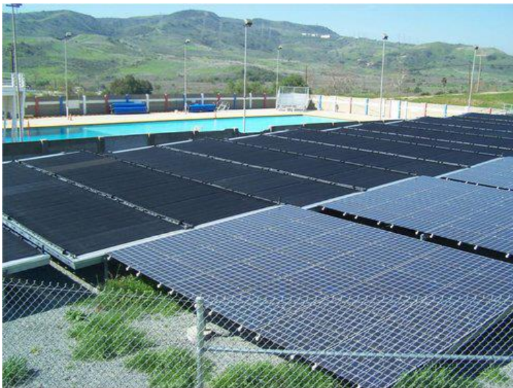
Figure 1: Solar pool heating system and solar photovoltaic system at Camp Pendleton, CA. 10 (8)
