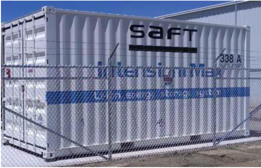
Figure 3: The large battery storage system at Fort Hunter Liggett. 11 (9)
