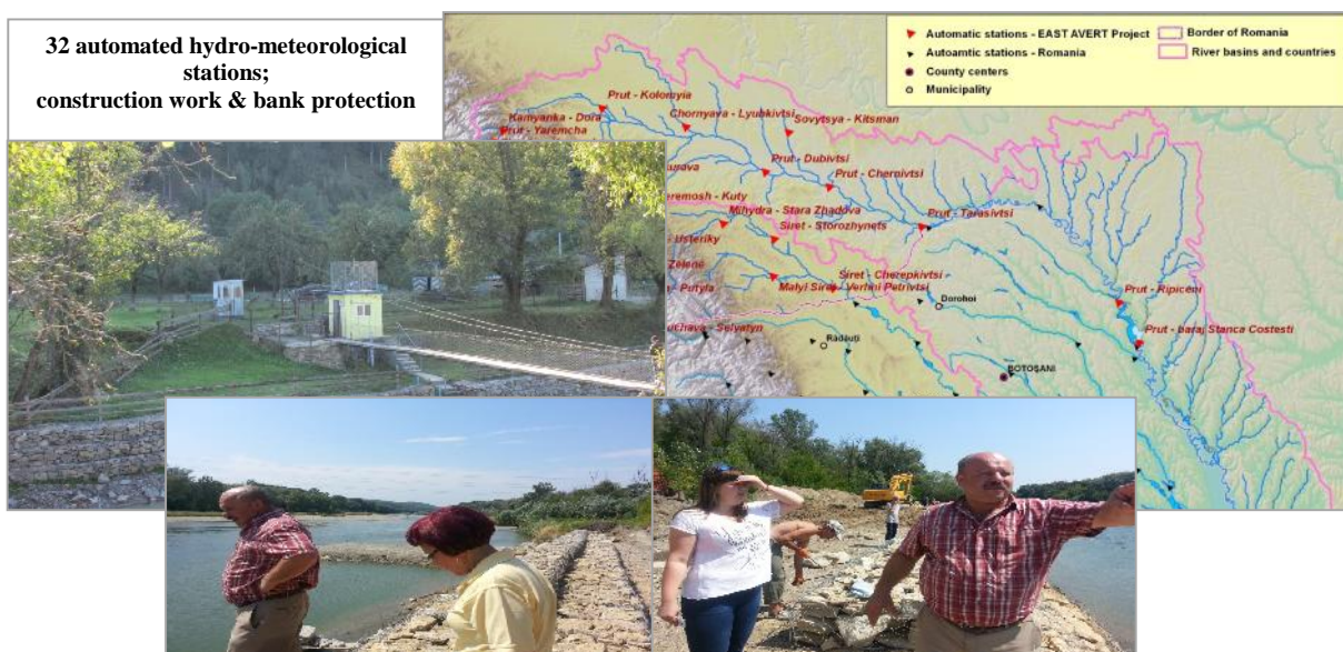
Figure 4. Instalment of 32 automated monitoring stations in the upper Prut & Siret River Basins (border region between Romania & Republic of Moldova (2 stations) and Ukraine (30 stations); works & bank protection for flood on the Ukrainian side
