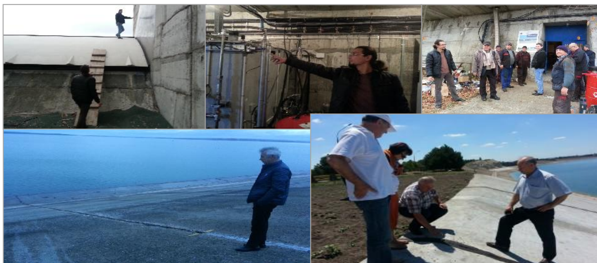
Figure 3. Enhancing the main hydraulic infrastructure on the Hydro-technical Complex “Stanca-Costesti”: installing new dam equipment for water level discharge control; rehabilitation works of the reservoir dam for prevention and protection against floods and accidental pollution events
