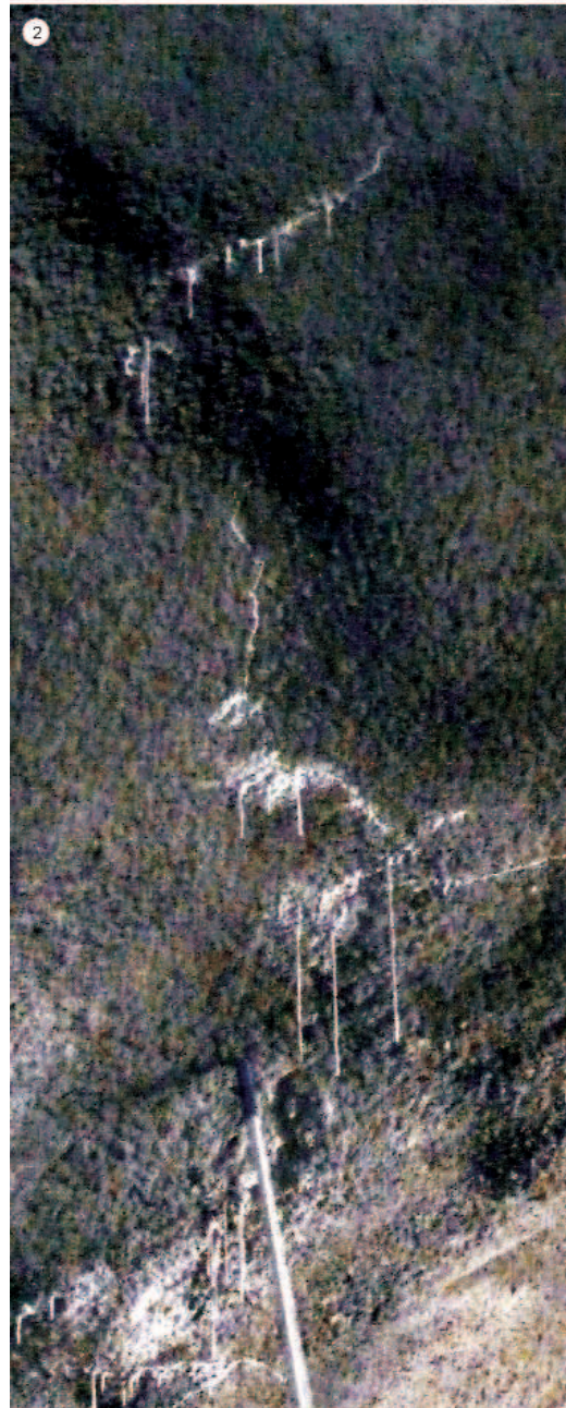
Photos 1–2. Precipitation of lime and dripstone along an open fracture (Interconnecting Passageway 3)
