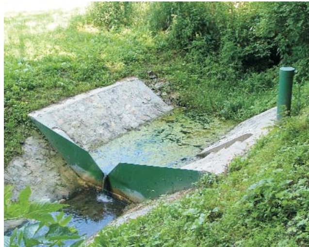
Figure 5. Picture of an overfall ( B10 ) – the concrete engineering structure with a Thompson overfall edge and water meter
