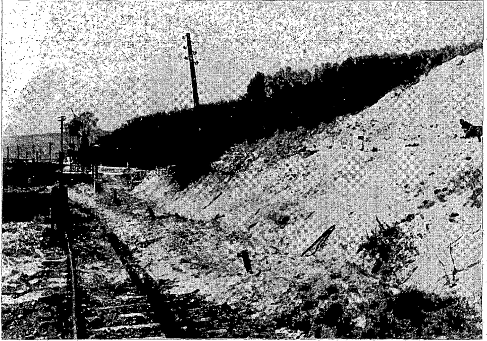
Fig. 8. The railway line section between Balatonkenese and Fűzfő damaged by the landslide of 1942, and a view of the zone of sliding by sections 419—421 (after L. LÓCZY JR.)
