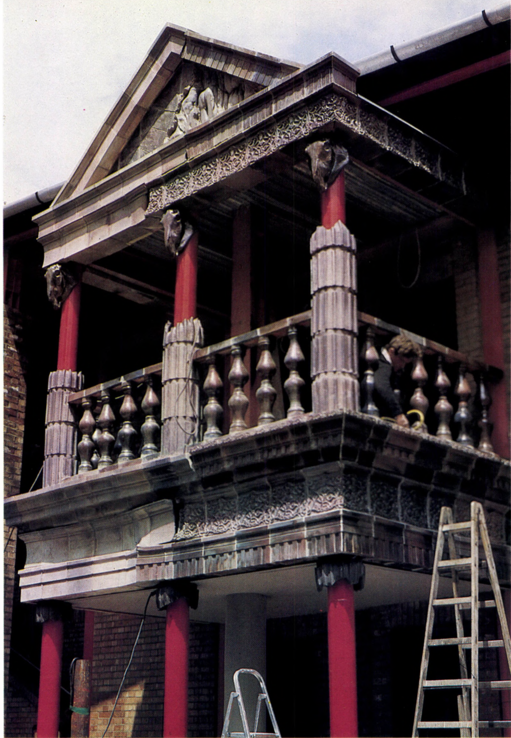
IMRE SCHRAMMEL: THE FAÇADE OF THE ENCHANTED CASTLE IN THE BUDAPEST LUNA PARK. 1987. SALT GLAZED CHAMOTTE, 77 Sq. m.
